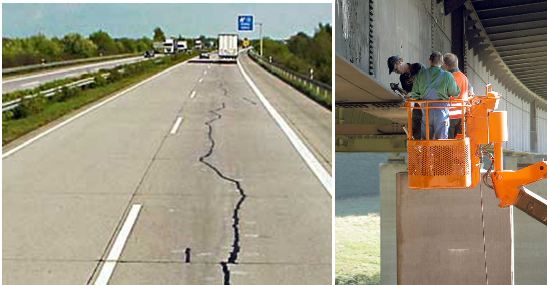
Figure 4: Examples of road infrastructure deterioration (Source: www.strassen.nrw.de ).
